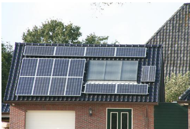
Figur 2-27 Building Adapted PhotoVoltaics (BAPV). Figuren viser et typisk takmontert PV-anlegg. Kilde: riddersolar.com
