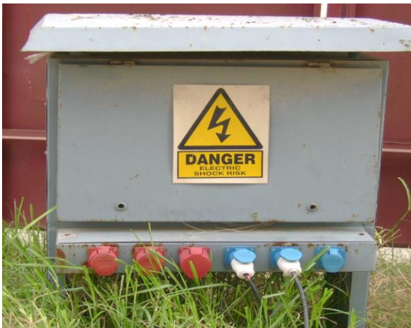
sign of danger was present at high voltage of electric panel
