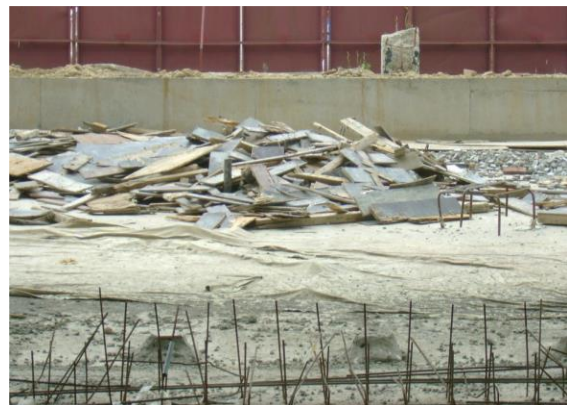
Improper soft/solid waste management on construction site
