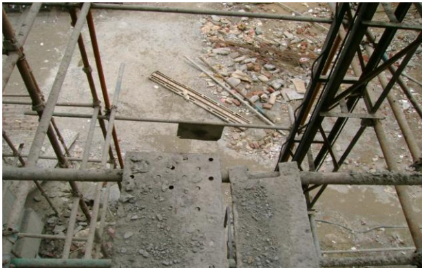
hazard can occur on site
