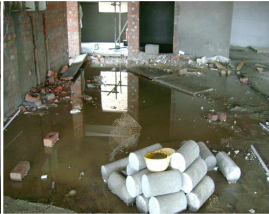
Presence of water on floors can cause accidents
