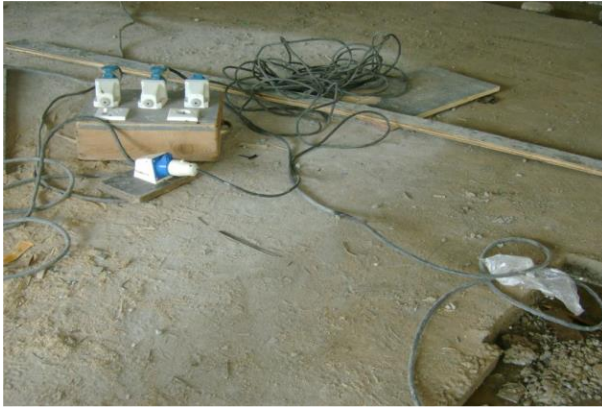
Unprotected electric connection can set fire
