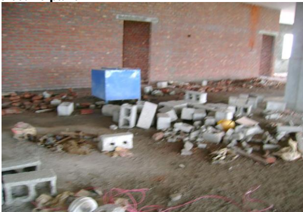
Presence of hard waste in the basement
