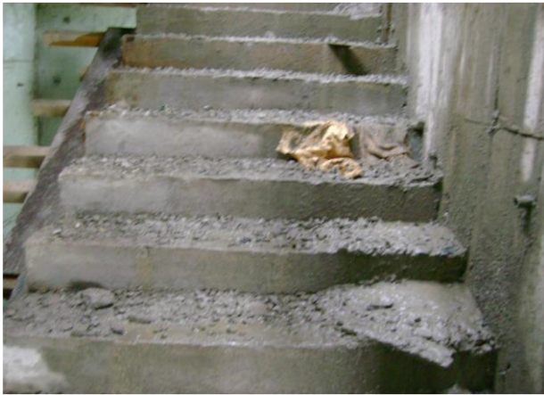
Unprotected stairs can cause slips
