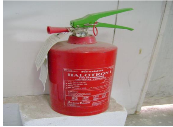
Fire extinguisher was present at the site
