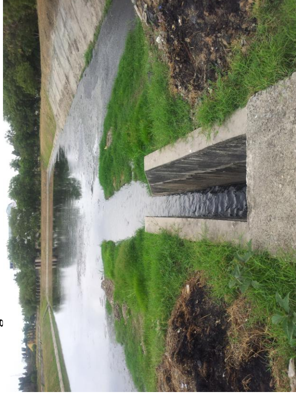
A Mikochei waste stabilisation pond in a state of disrepair
