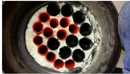
(f) The space between the small pipes where foamed to keep them together.
