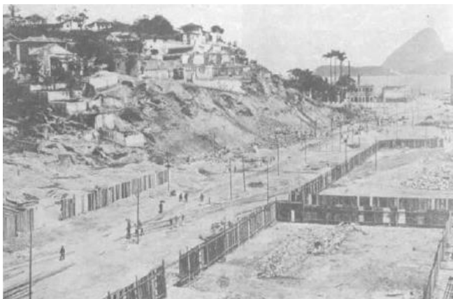
Ground of Avenida Central and hillside of Morro do Castelo in 1905. The Mountain was entirely removed in 1921 (Benchimol 1990)
