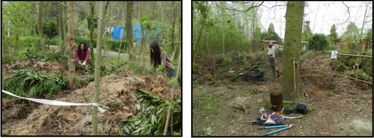
Figure 5: Left: This researcher and one DZ resident helping to construct branch walls for Compoststraat (Photo credit: DZ resident). Right: The challenge of an overabundance of organic waste that is not separated.
