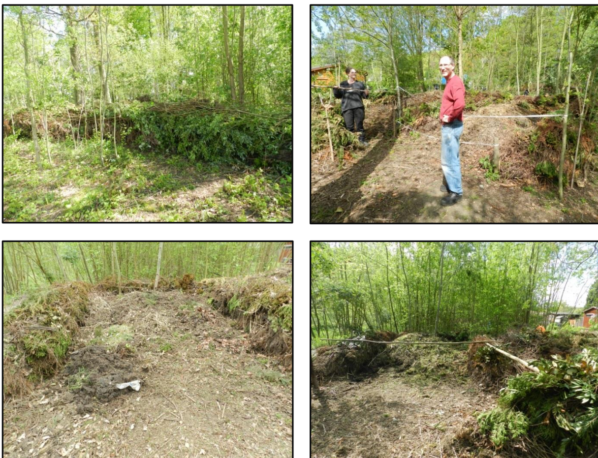
Figure 13: Photographs showing wall structures and compartments made by Roos and DS volunteers to separate organic waste.
