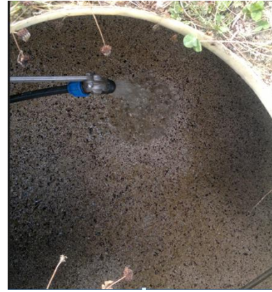
Fig. 8c: Nozzles in P-filters at Høyås treatment system.
