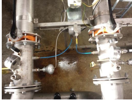
Figure 66: The small, blue pipelines are connector to the pressure transmitter in the middle, and to the main piping to the left and right.
