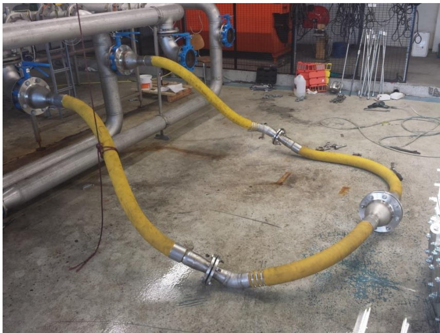
Figure 18: The connecting hoses, connected to each other to create a closed circuit of flow, to measure the systems internal pressure drop.
