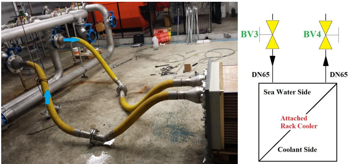
Figure 25: The yellow connecting hoses installed to the rack in a 4-pass configuration. The blue valves are visible at the other end of the hoses, and the arrows represent the flow direction. To the right is the flow chart symbol.
