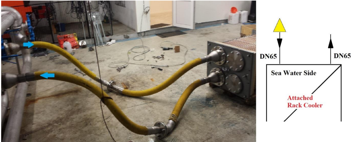
Figure 20: The yellow connecting hoses connected to the rack in a 2-pass half rack configuration. The blue arrows represent the flow directions in the hoses. To the right is the situation represented in flow chart symbols.
