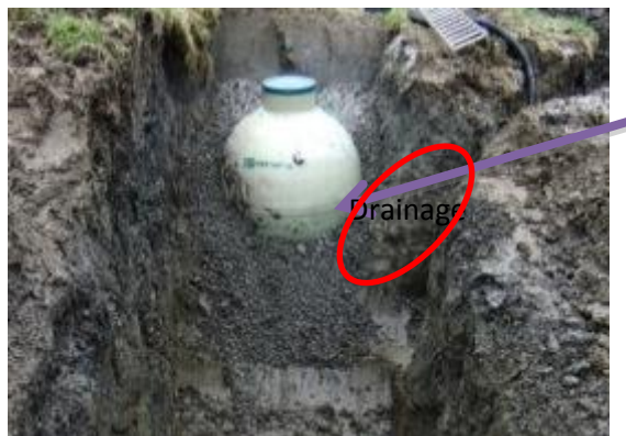
Photo: 5 Pumping chamber covered by gravel
