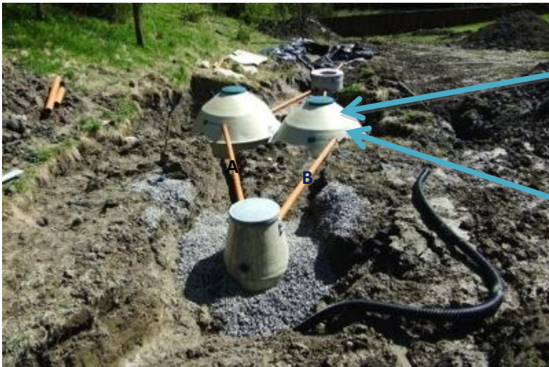
Photo: 15 Pipe fitting arrangements for phosphorus filters
