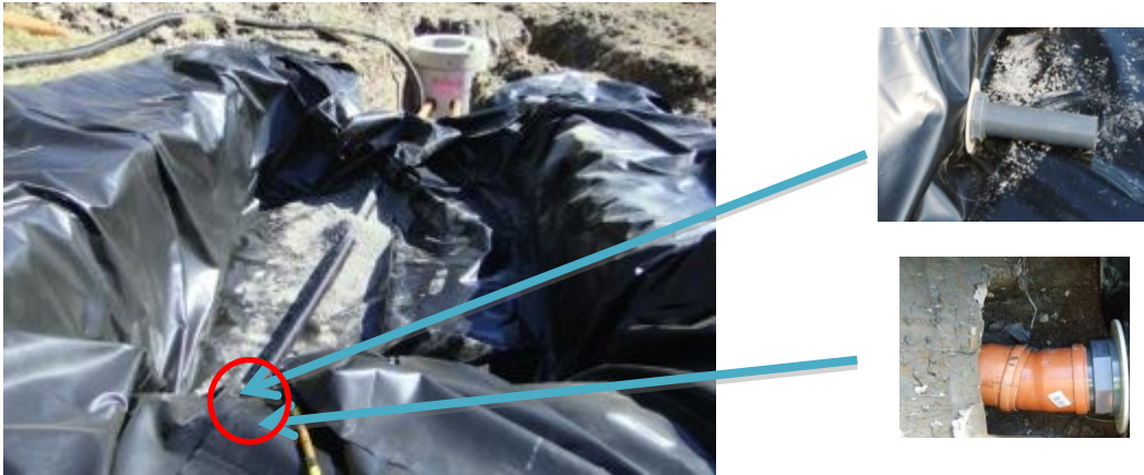
Photo:20 Non permeable membrane covering sand filter trench and outlet pipe fittings arrangement
