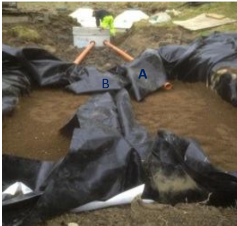
Photo: 21 Two compartment sand filter; one compartment for each phosphorus filter tanks
