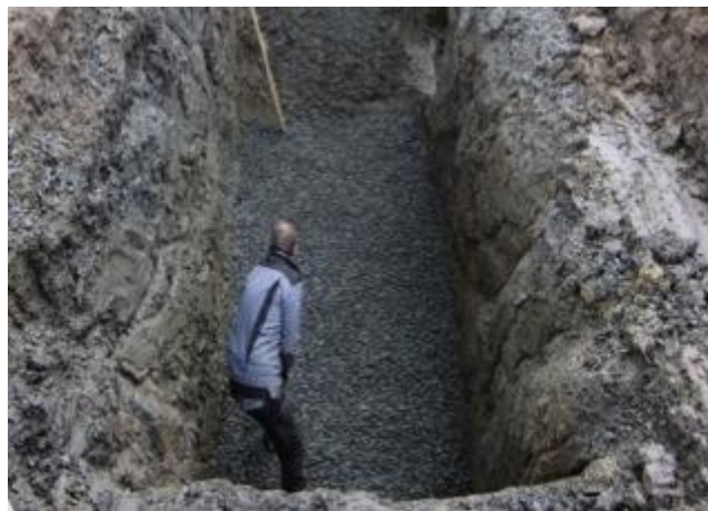
Photo: 2 Leveling gravel in a trench as base material for septic tank
