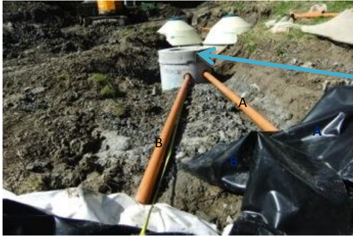
Photo: 16 Inspection and sampling chamber
