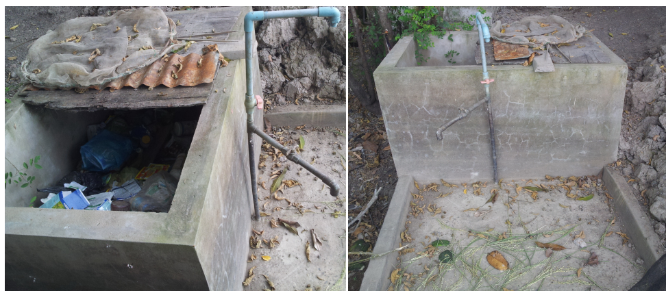
Figure 11: The separate area of mixing pesticides and destroying pesticide packages safely
