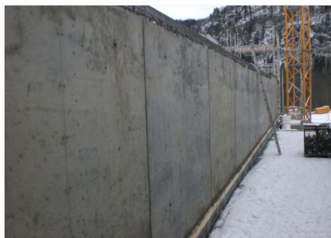
Figur B.6: Overflate - standard betong [1]
