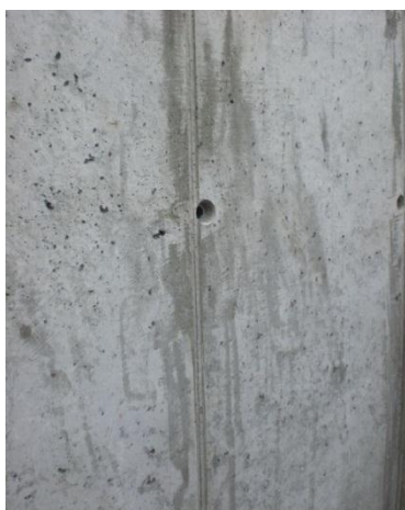
Figur B.5: Overflate - standard betong [1]
