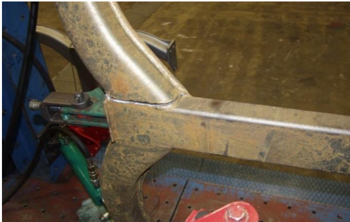
Figure 1.2: In this illustrated case, the crack is caused by horizontal and part sideways forces on the plough beam. This creates tensional stress on both the front and the side of the beam. The crack growth is appearing at the welded intersection between the leg and the main tube of the beam. This is not very surprising, since the area is subject to the highest bending moment, and crack growth is then made from the micro cracks around
