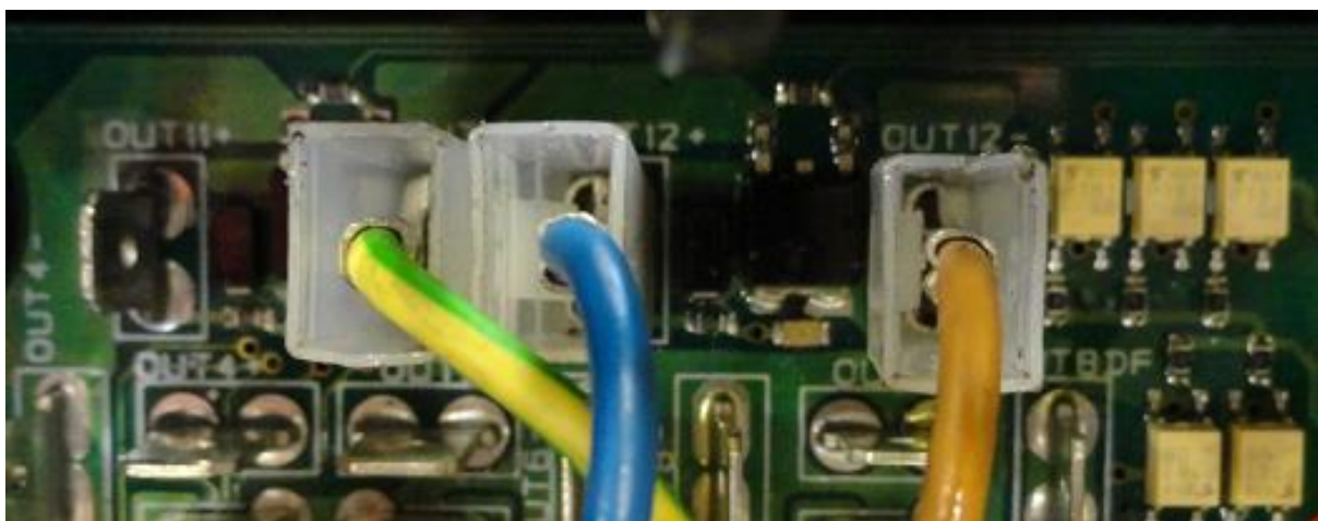
Figure 8.11: The signal output cables for the directional valve control were connected onto the printed circuit board according to the instructions following the software delivered by Kverneland Group Mechatronics. Illustration by own photo.
