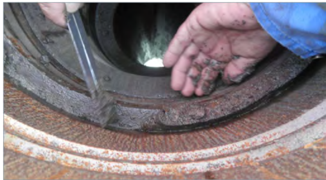
Figure 301: Cause of failure: lots of debris trapped between spool landing shoulder and TH. [2]
