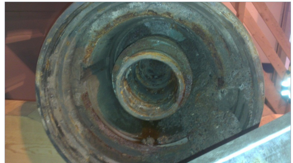
Figure 313: Corrosion issue on TH. [2]
