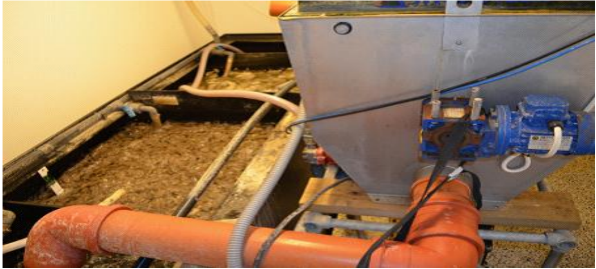
Figure 3.4 Water treatment room.
