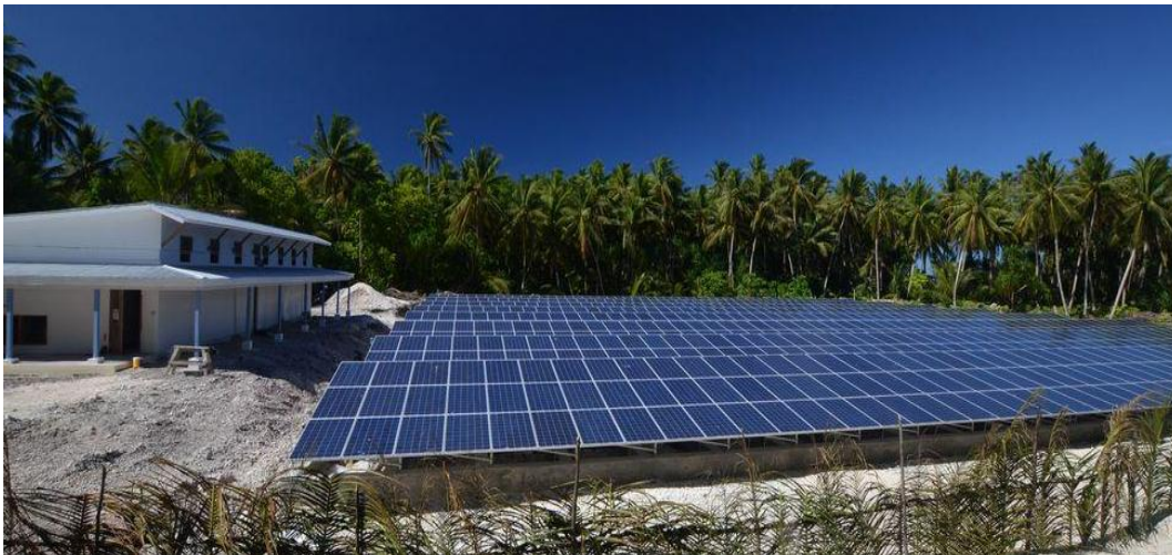
Figure 28: PV array of Atafu mini-grid. [15]
