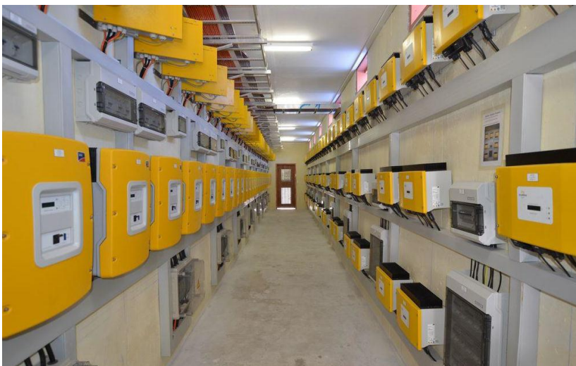
Figure 27: The inverter room of the Atafu plant. [15]
