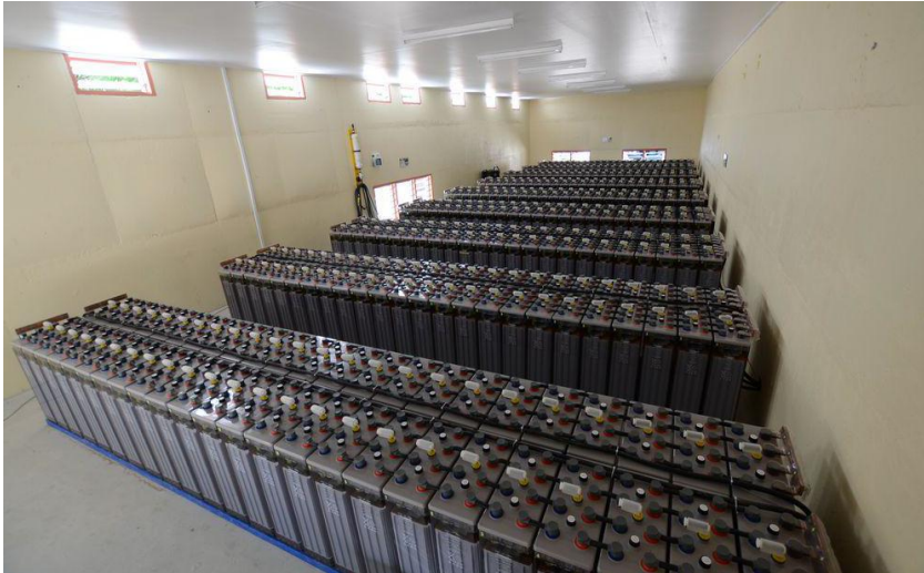
Figure 26: Battery bank of Atafu mini-grid. [15]
