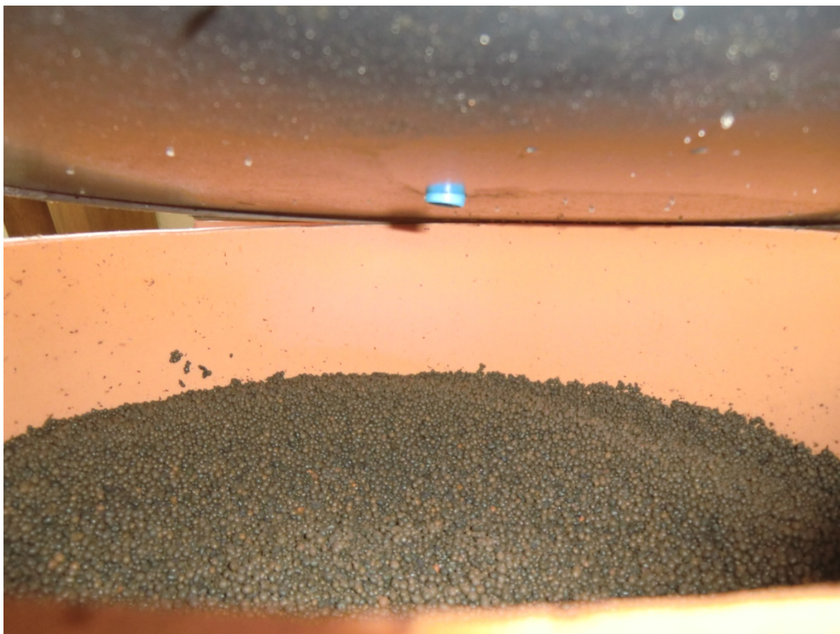
Figure 4: Filtralite® inside the filter, with the nozzle in the lid.
