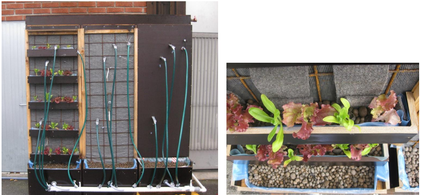
Figure 3 – Completed filter wall (left) and detail of planter shelves with felt strip irrigation system (right)
