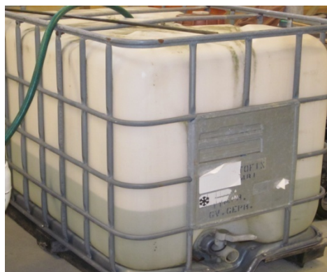
Figure 7: Arsenic contaminated reject water collection tank.
